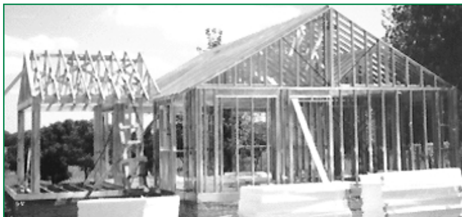
Steel-framed construction is expanding the role of steel in residential and light commercial construction.
