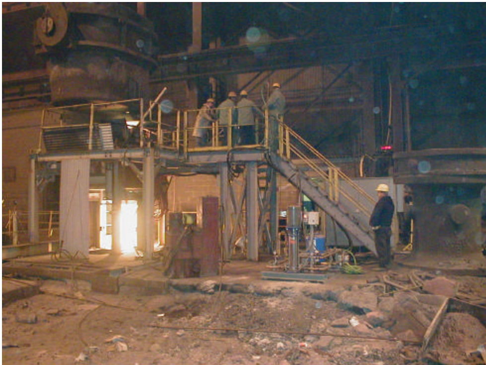
Figure 4. Overall view of the test site from across the plant's aisle during a pouring test.
