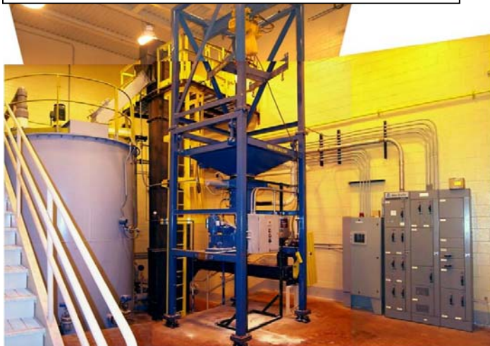
Figure 5: Mixing and Conveying Equipment
